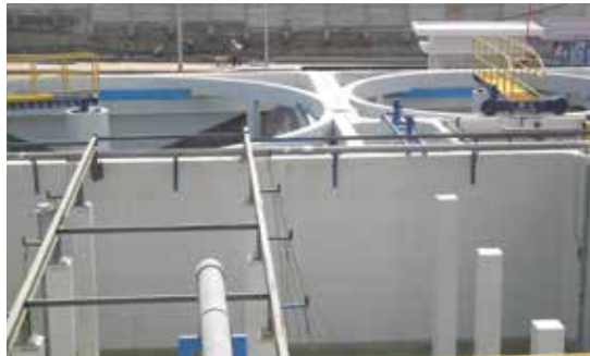
Indolakto New East waste treatment plant East Java, Indonesia
