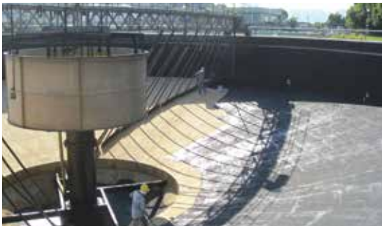
Sewage treatment plant, sedimentation tanks Yuen Long, Hong Kong
