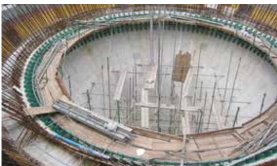
Sludge tanks at Changi Water Reclamation Plant Singapore
